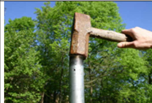
Drive wider pipe into ground (better to use a 2 x 4 between hammer and pipe)
